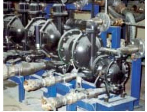
ARO diaphragm pumps transfer bases for paint formulation.
